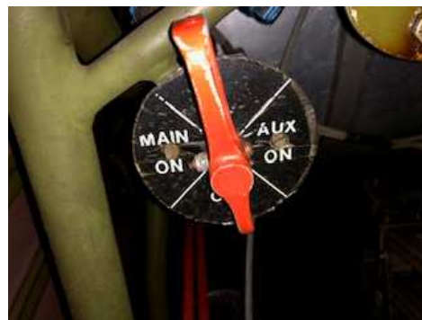
Fuel Selector presently in 'off' position Rotate 90 degrees counter clockwise To 'off'
